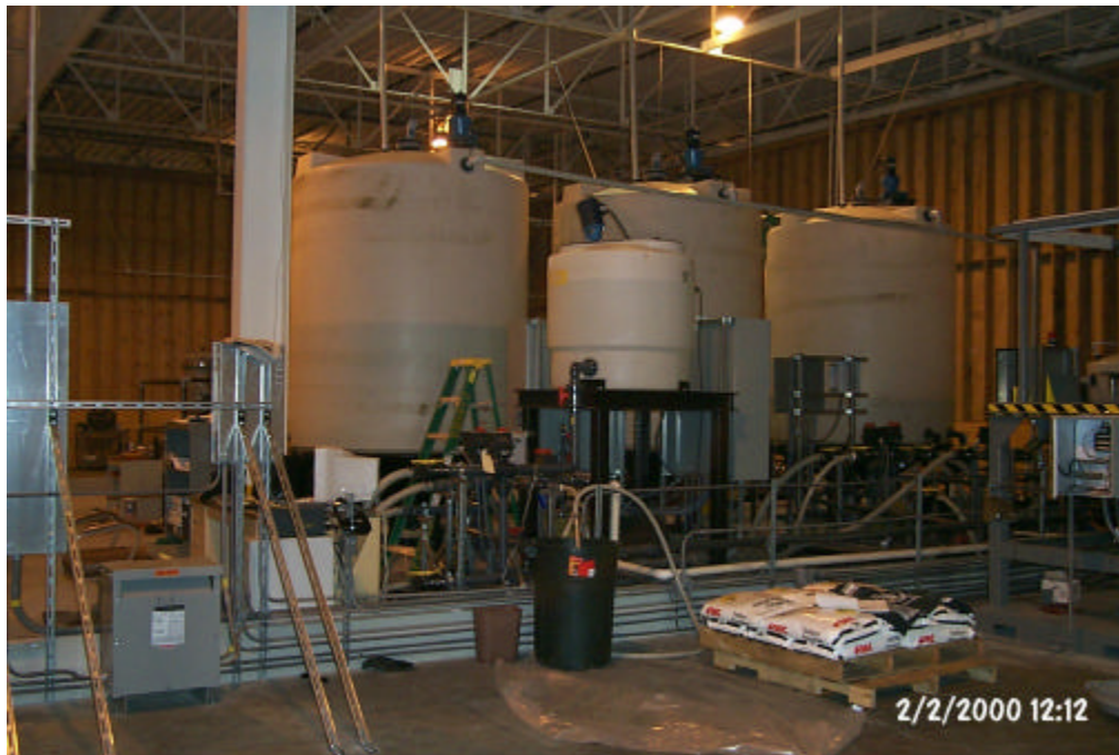
Figure 3-3: Picture Shows Oxidant Batching Tanks and Associated Piping for Oxidant Application (Marley et. al. 2003)
