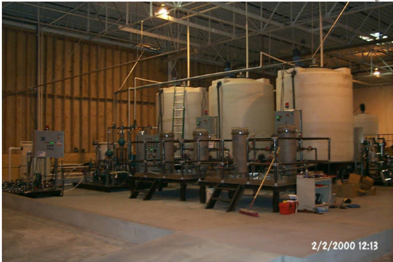
Figure 3-4: Picture Shows Dosing and Filtration Skids and Associated Piping for Oxidant Application (Marley et. al. 2003)
